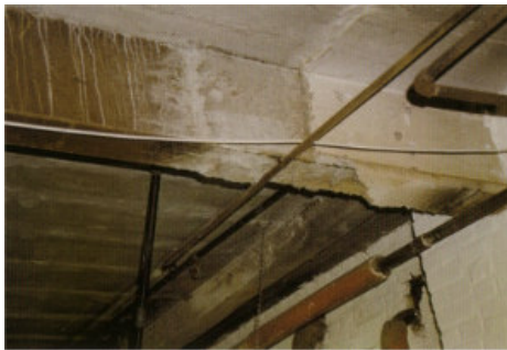
Steelwork coated with asbestos spray for fire protection. The photograph also shows a section of asbestos lagged pipework.
