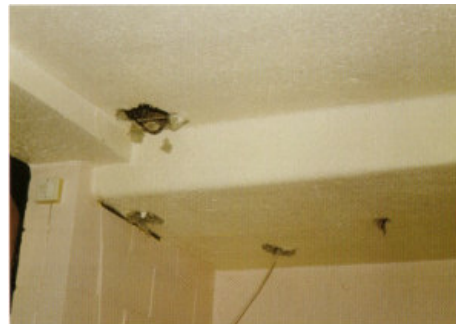
The insulation on both has been partly removed. A ceiling coated with asbestos spray, which has been damaged by building work.
