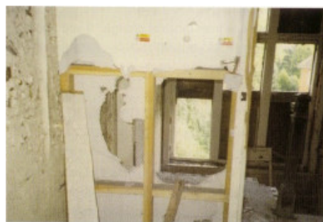
A severely damaged wall in a domestic premise made of asbestos insulation board.
